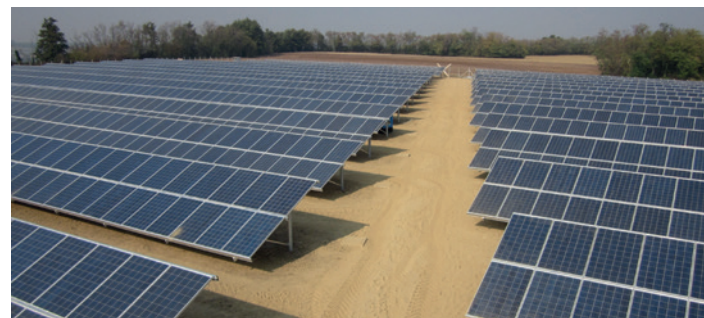
Park: Salmour, Italy Park size: 6,0 Mwp Mounting system: FMS V2
