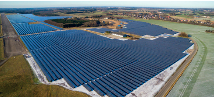
Park: Vandel, Denmark Parksize: 75,0 Mwp Mounting system: FMS-H4
