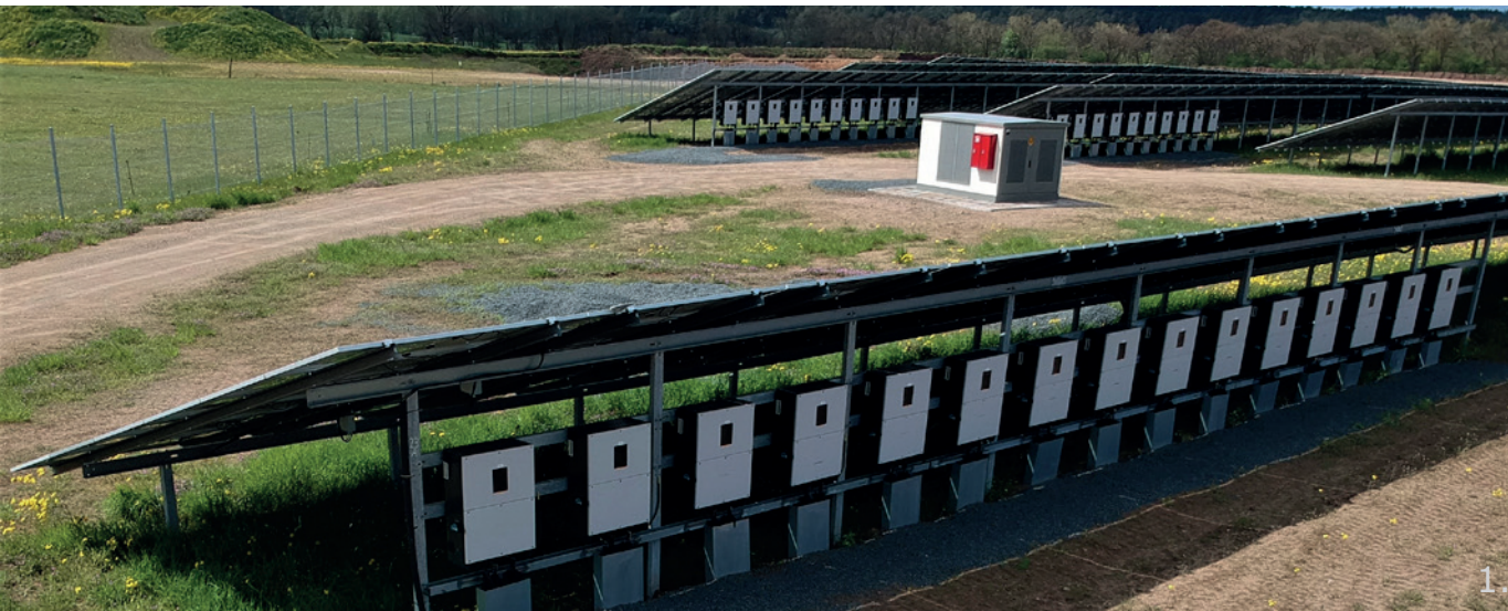
Picture 1: Easy & direct inverter mounting Picture 2: Drawing of inverter mounting Picture 3: Transformer station
