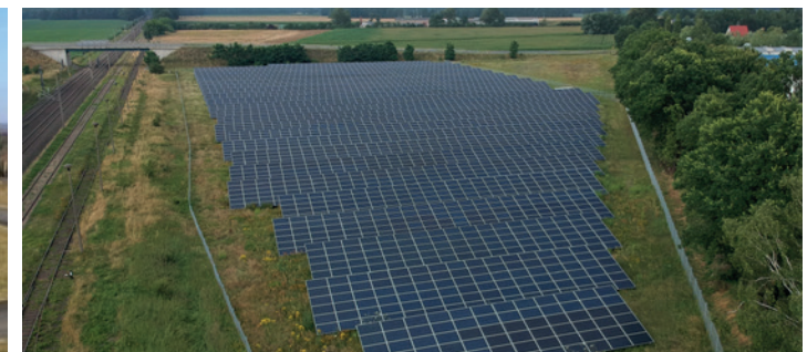
Park: Mainburg, Germany Park size: 25,0 Mwp Mounting system: FMS H6
