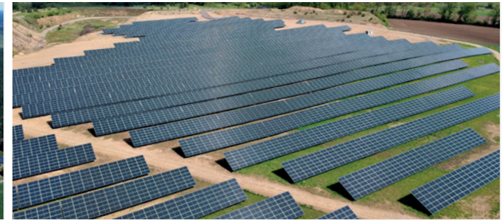
Park: Sophienhof, Germany Park size: 9,2 Mwp Mounting system: FMS-H6
