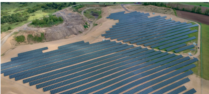
Park: Sophienhof, Germany Park size: 9,2 Mwp Mounting system: FMS H6
